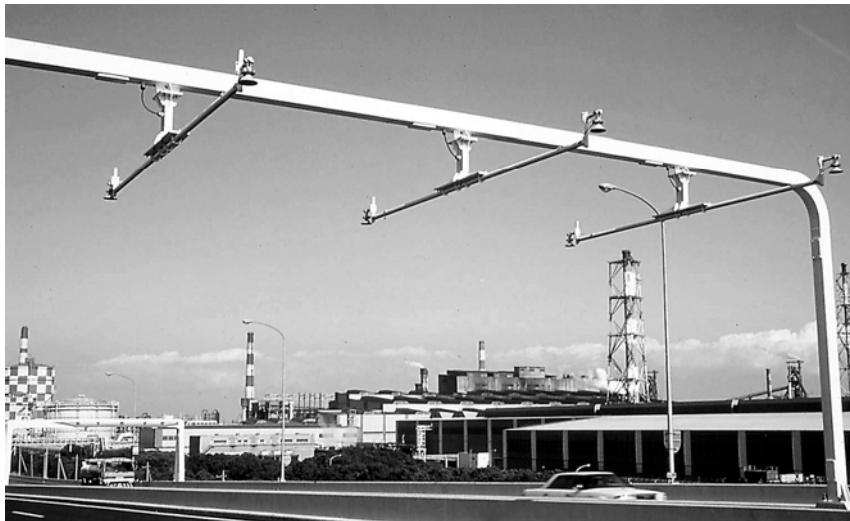
Fig.5.2. Overhead ultrasonic vehicle detectors (double node)
